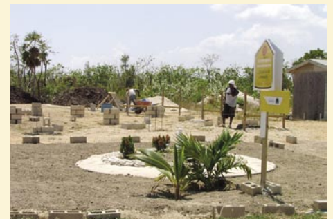
Houses demolished in East End to make way for rebuilding. (top) Foundation laid for one East End house that is undergoing rebuilding. (bottom)
